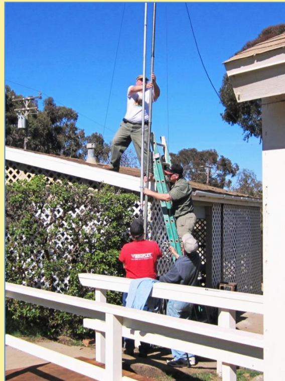
Above right: Installing the massive tri-band Yagi beam antenna took four guys, including Joe, NZ6L on the roof with Ray, N6HE; Dan, K6DPY; and Clay, AB9A.
