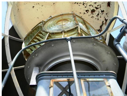
Above: In this 2012 photo the lantern room ceiling at Pt. Vicente Lighthouse shows extensive peeling paint, while iron railings outside (not shown) have extensive corrosion from marine air. These conditions highlight preservation needs for many lighthouses throughout the world. PHOTO: AI6DF
