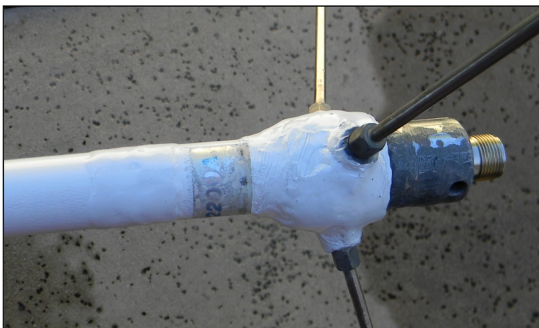
Figure 7. Antenna bottom section after reattaching/reinserting internal antenna components; and, applying medium texture fiberglass cloth, two-part epoxy and white spray paint (after strategic placement of masking tape) to reconstruct the antenna at the two saw cuts and complete the repair.
