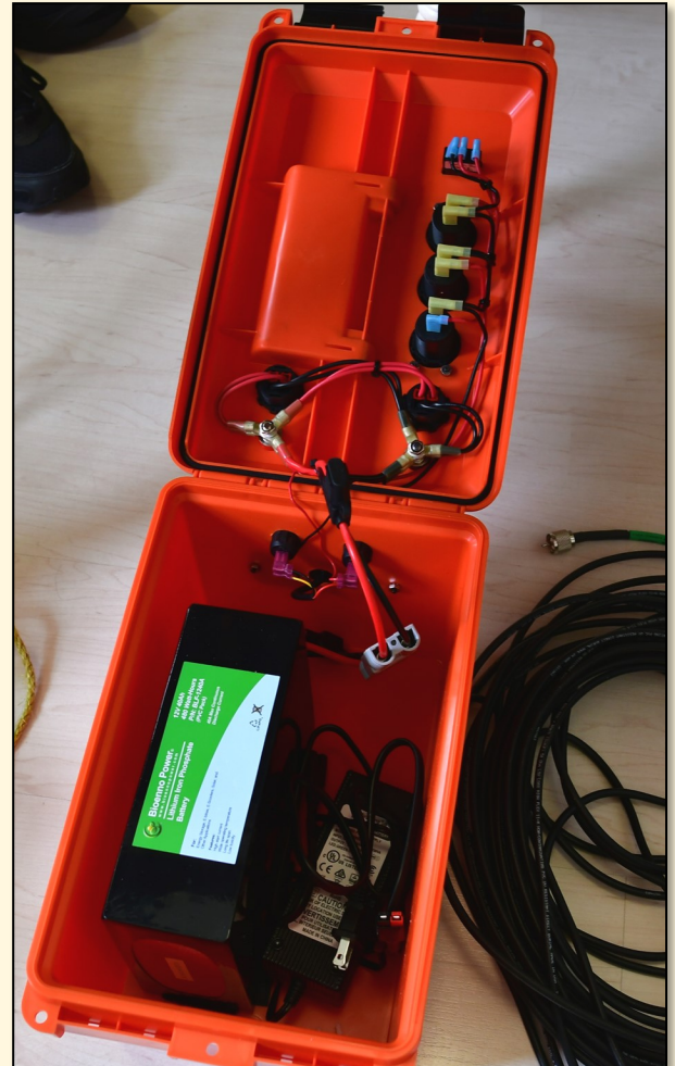
Above: A 40 Amp-hour lithium iron-phosphate battery being set up under the kitchen table for 2020 home Field Day operation entirely on portable power. PHOTO: DIANA FEINBERG, AI6DF
